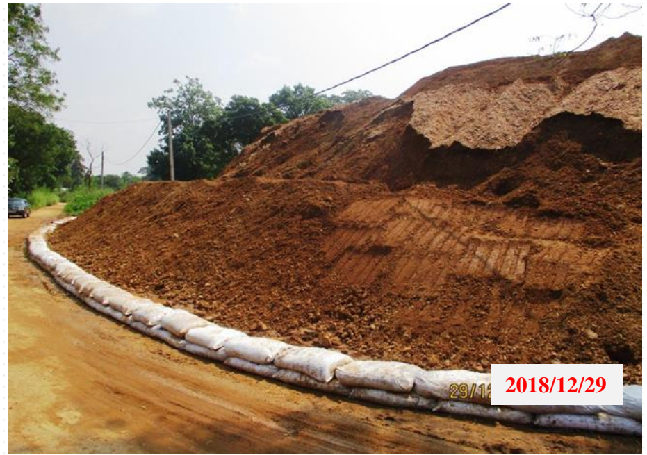
Protection dam to prevent mud flow to private land UMO 022 CH. 5+160 (RHS)
