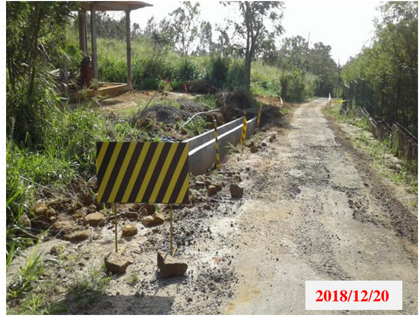
Line drain UBA- 076 CH. 0+418 (LHS)
